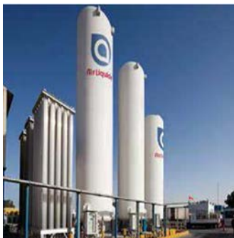
Liquid Oxygen Supply System
