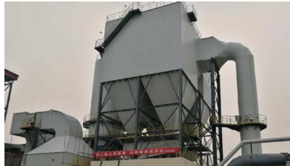
Project of Desulfurization and Denitrification of Flue Gas for 58MW Chain Boiler of Shandong Yanzhou Juyuan Thermal Electricity
