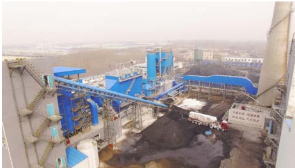
Project of Desulfurization and Denitrification of Flue Gas for 58MW Chain Boiler of Shandong Yanzhou Juyuan Thermal Electricity
